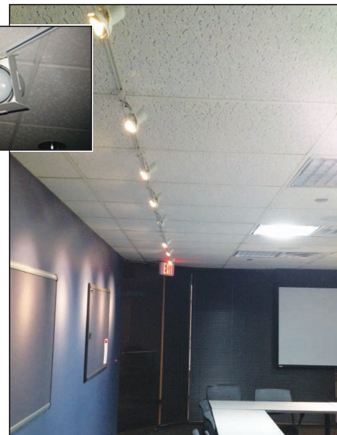
In its offices — but especially in its conference rooms (left and right) — DNV GL replaced outmoded light fixtures (above) and installed new state-of-the-art induction, LED and LWHP T8 fixtures throughout the suite.
